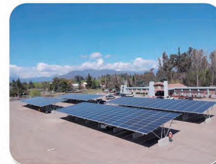
500KW SFS-CP-03 Commercial Carport mount (Chile)
