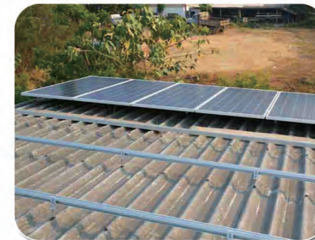
500KW SFS-PR-01 Asbestos Roof Mount(Thailand)
