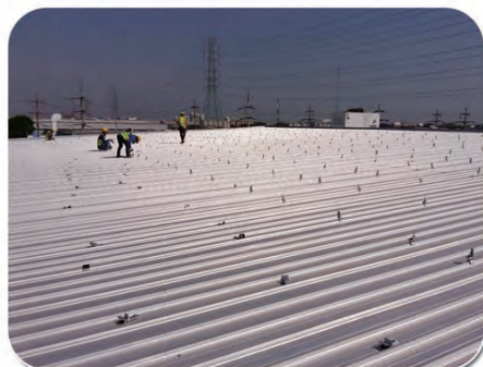
1MW SFS-PR-01 Tin Roof clamp mount (Thailand)
