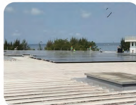
900KW SFS-PR-01 Tin roof solar mount (Vietnam)
