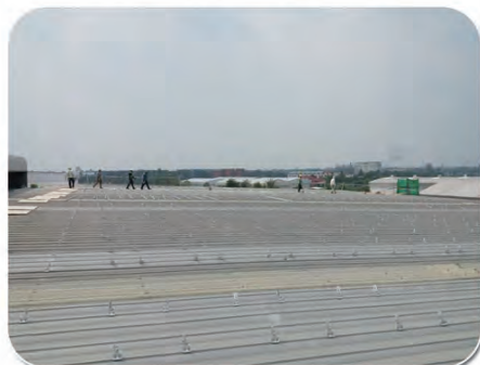
2.5MW SFS-PR-01 Tin roof clamp mount( Thailand)
