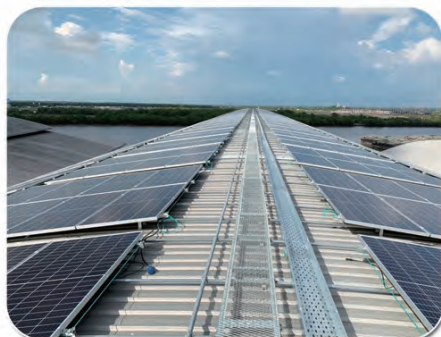
1MW SFS-WW Walkway mount System (Thailand)
